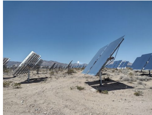
Heliostats in Ivanpah Solar Field, Unit 1
